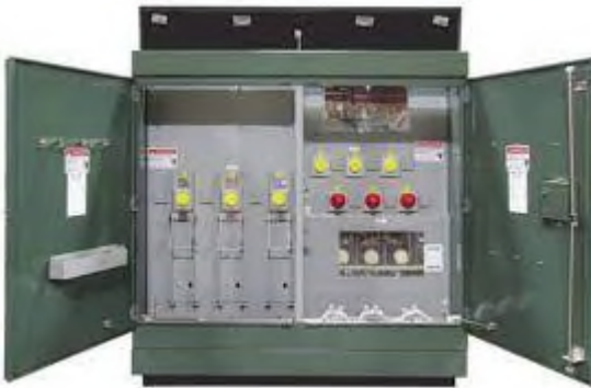
Open pad-mounted switchgear
