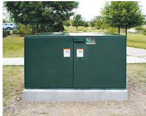
Closed pad-mounted switchgear on vault
