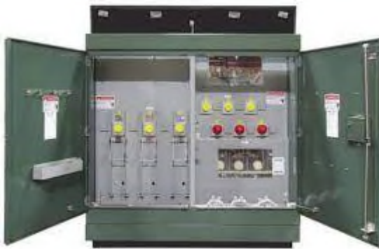
Open pad mounted switchgear
