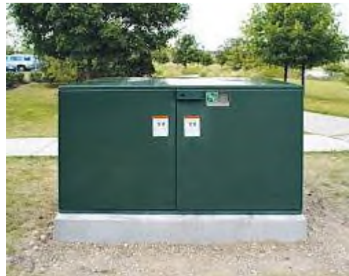
Closed pad mounted switchgear on vault
